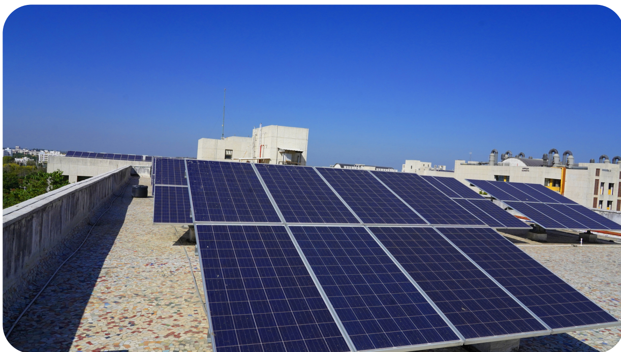
Roof top solar panels (345KWp)
